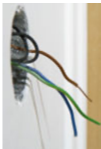
Exposed electrical wires.
